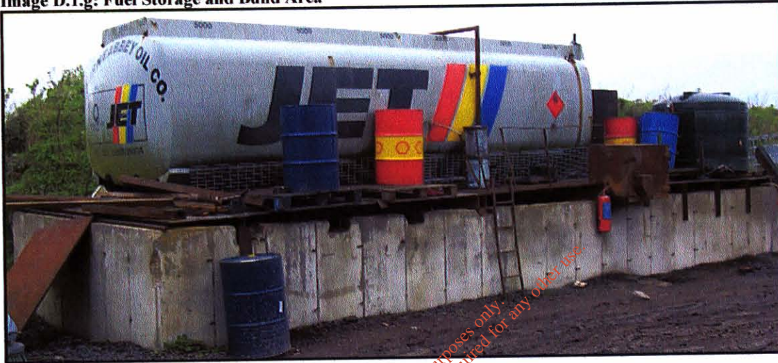
Image D.1.g: Fuel Storage and Bund Area
