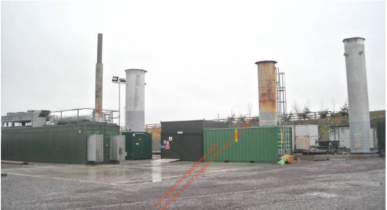
Plate 2-6: Landfill Gas Compound
