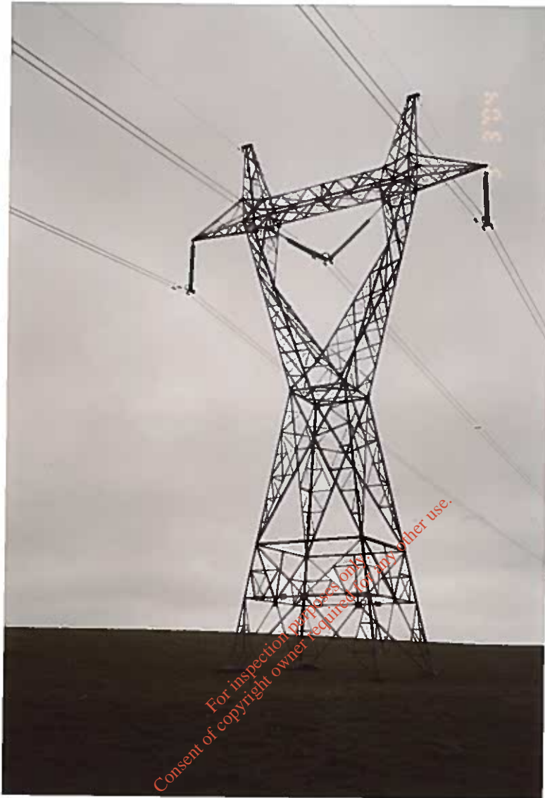
400 KV PYLON. PYRAMID OF UNDISTURBED GROUND TO BE RETAINED AT ITS BASE.
