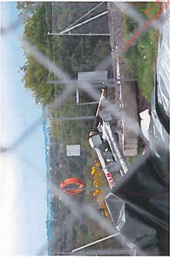
Agitator used to treat/ keep fresh the wastewater in the lagoons
