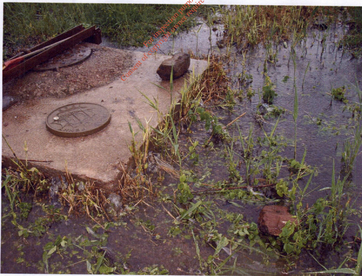
Biscuit lifted sewage pouring out
