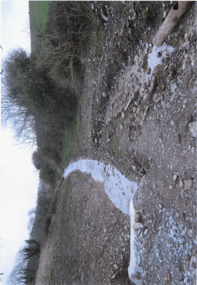
GLANAGOW WATERCOURSE EX BOARD GAIIS (WIPP) SOUTH DIRECTION
